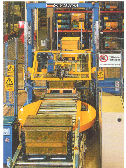
Fully automatic strapping installations
